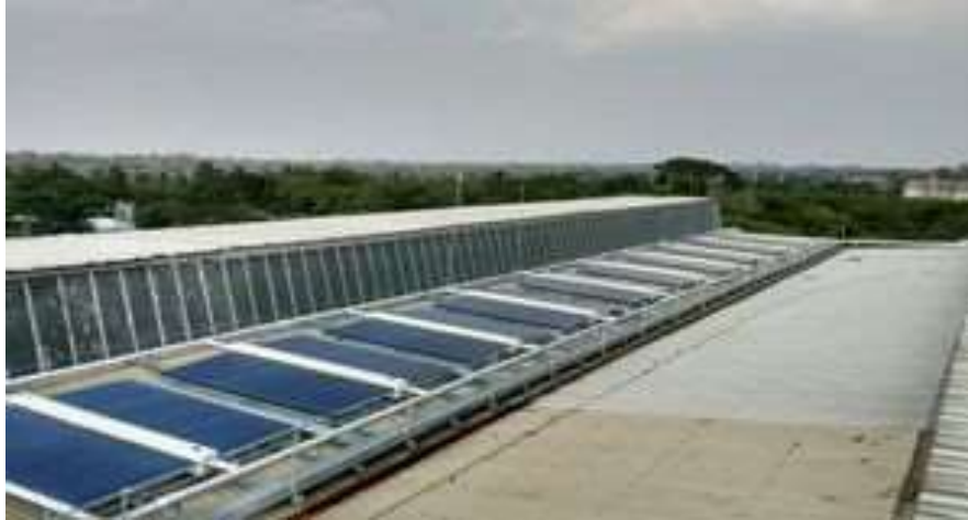
Figure 12. 360 kW th solar thermal plant for transportation industry in India (INTEC, 2015)
