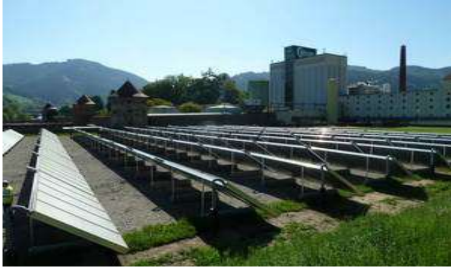
Figure 10. 1,064 kW th solar thermal plant for beverage industry in Austria (INTEC, 2015)
