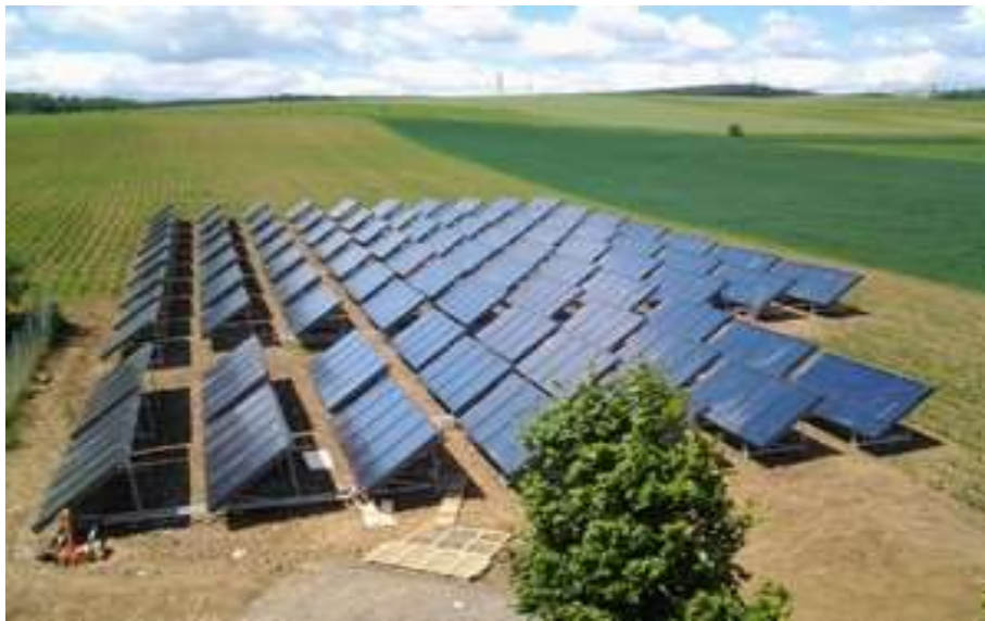
Figure 8. 746.9 kW th solar thermal plant for meat industry in Austria (INTEC, 2015)
